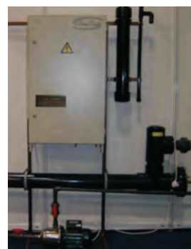
Fig. 1. Ozone generators with barrierless electrode system
