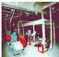
General view of the facility to prepare water-coal mixture
